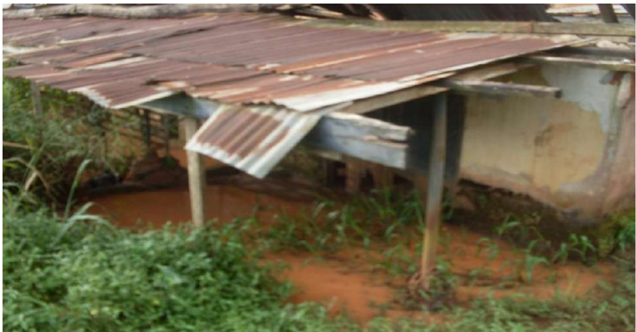
Figure 10. Abandoned residential house in flood area.
